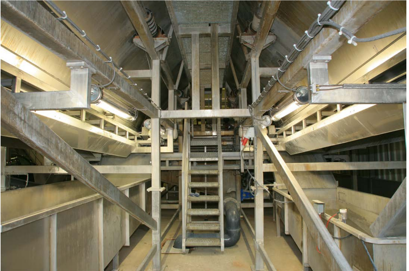
Wastewater treatment plant, HAK, Netherlands
